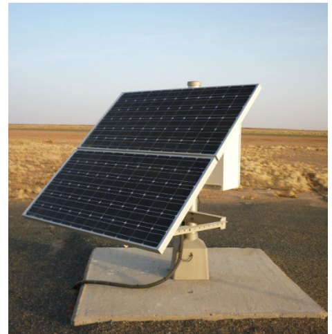
Existing solar array and concrete pad, retained for the new system
